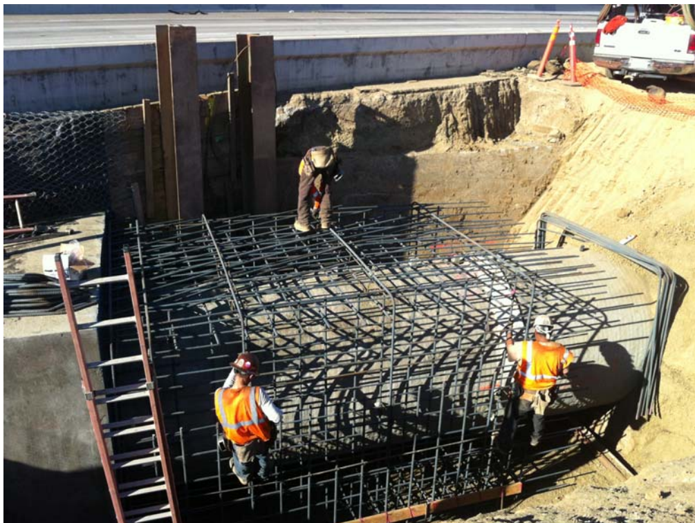
July 27, 2012. Installation Of Reinforcement Steel for 2 nd Segment of Mokelumne Aquaduct Encasement
