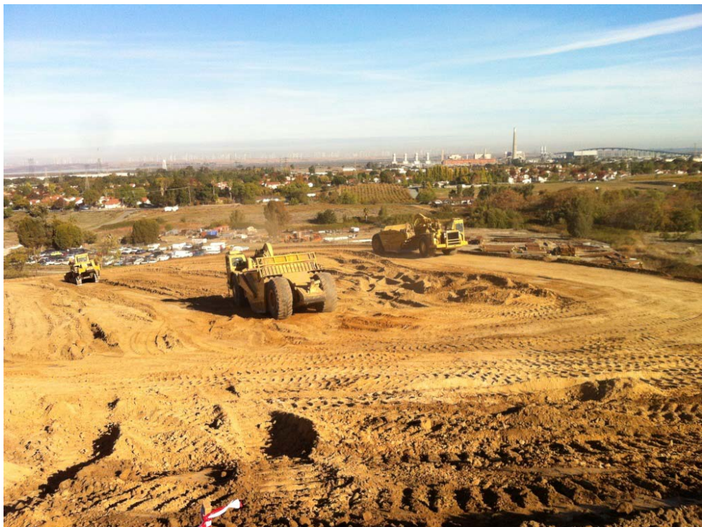
04SF-120 Nov. 13, 2012. Cut and Fill Earth Moving Viewed From Top of Hill
