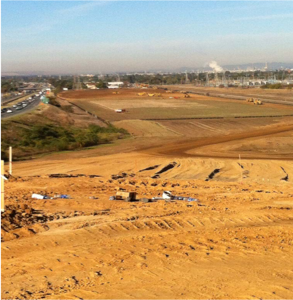
04SF-120 Nov. 12, 2012. Cut and Fill Earth Moving Viewed From Top of Hill
